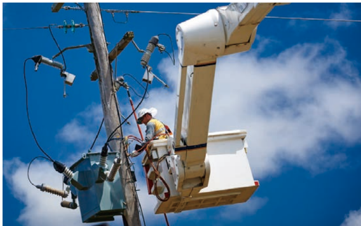
Victoria Power Networks is the holding company of electricity distribution networks, Powercor and CitiPower.
